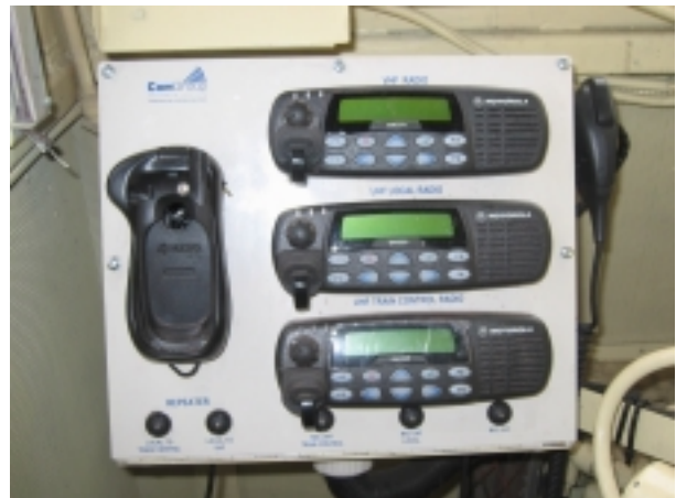
Figure 3 - CDMA telephone cradle and mobile radio transceivers on an ARG locomotive
